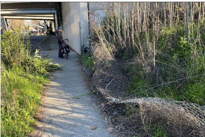
Broken fence, overgrown weeds on Olive Street south of underpass
