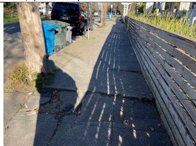
Cracked sidewalk on east side of Olive Street between Hazel and Sebastopol Ave.
