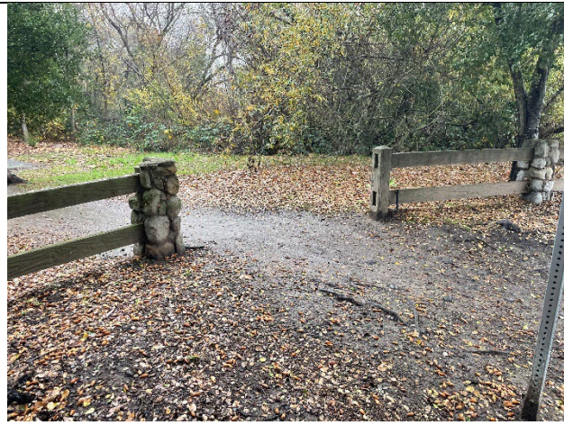
Another view of mud resulting from gap in pavement
