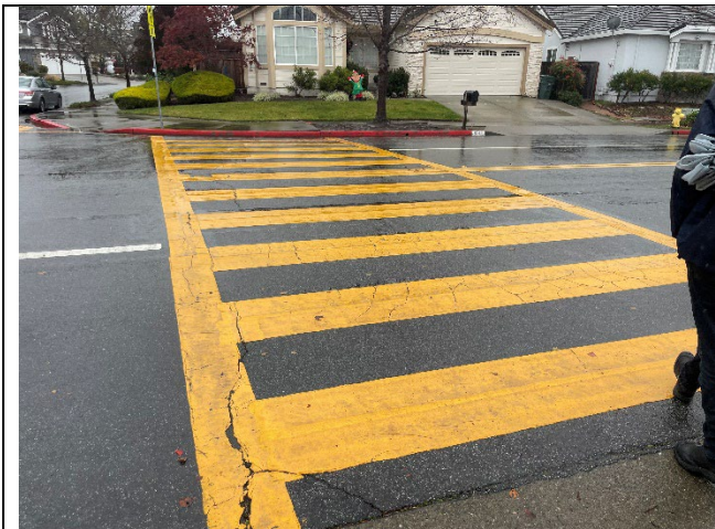
Crosswalk at Hartman and Quarry (missing curb ramp)
