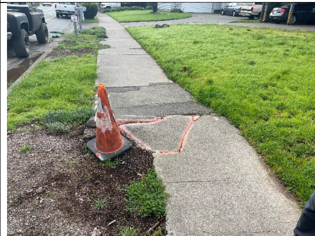
Damaged sidewalk on W. 3 rd
