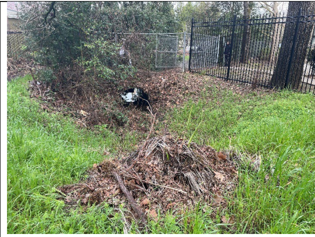
Example of one of the tunnels/culverts near walking path that participants expressed concern about.
