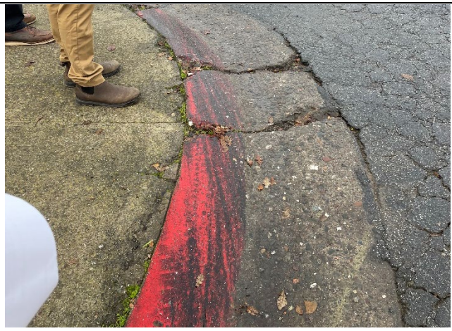
Evidence that drivers “cut curb” at Ellis & Madison.
