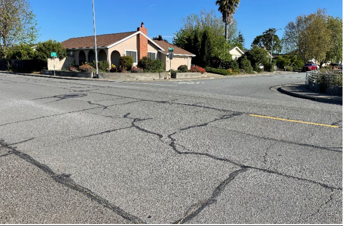
Intersection of Ponderosa Drive & St. Francis – no curb ramps (or painted crosswalks for that matter)
