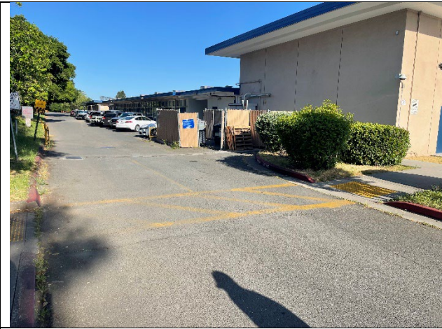
Faded crosswalk at entrance of staff parking lot across school driveway. Can use thermoplastic here, if able.
