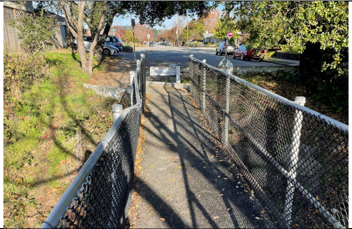
Franquette foot bridge, difficult for bicyclists to cross, bent railing
